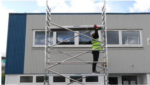
15. Fit your working platforms on the 5th rung down from the top of the tower.
