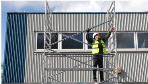
15. fit your additional diagonals to continue the bracing pattern. Running off the rung of your last brace.
