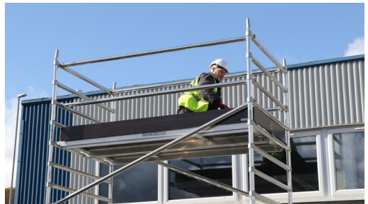
18. Correctly fit toe-boards as shown in the images.
