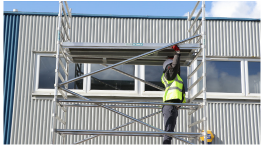
16. Fit your working platforms on the 5th rung down from the top of the tower.
