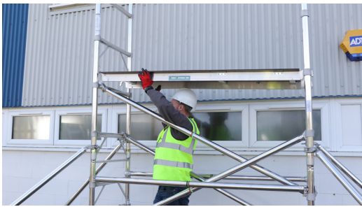
11. From the temporary platform, fit 1 diagonal brace to 3rd rung down and fit trapdoor platform over the hook. Offset platform to oneside.
